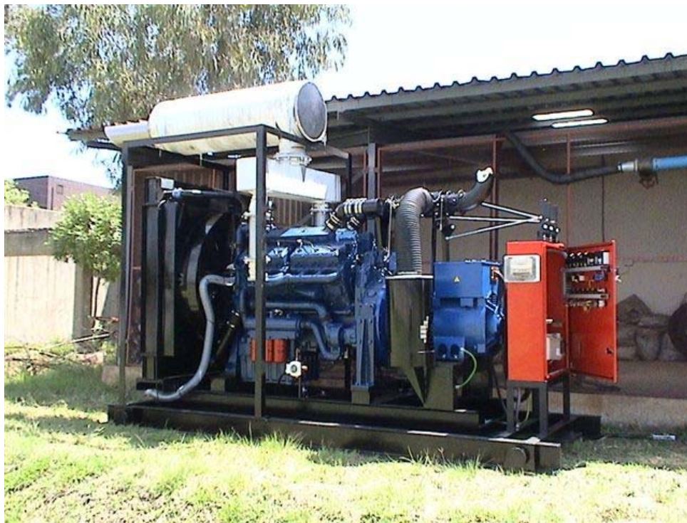
Figure 4. The gas engine coupled to a 150kVA synchronous generator.
