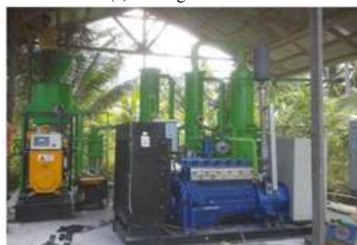
(b) Downdraft gasifier & gas engine 50 kW has installed at PLN in Indonesia
