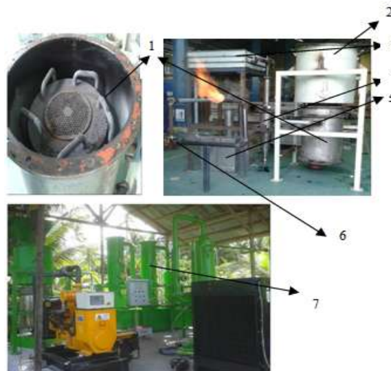
Description : (1)Reactor, (2) Biomass tank, (3)Cooler, (4)Cyclone, (5)Filter, (6)Blower, (7)Wet scrubber Fig. 7. Downdraft machine gasification
