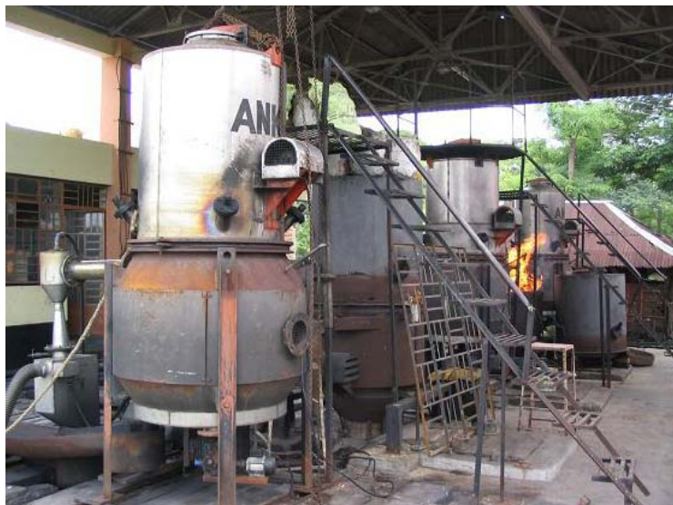
Figure 9: 5 x 100 kW biomass gasifier at Gosaba Island, West Bengal, India. (Source: Abe, 2005)
