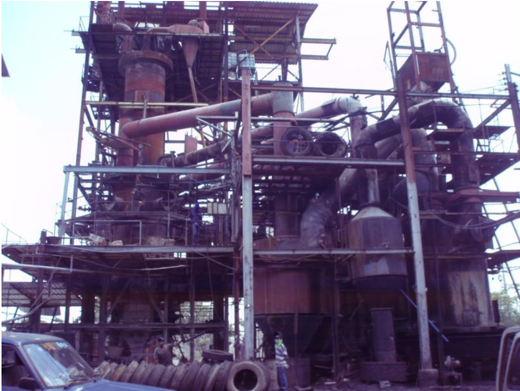
Rubber gasification plant at Lime Minerals, Saraburi
