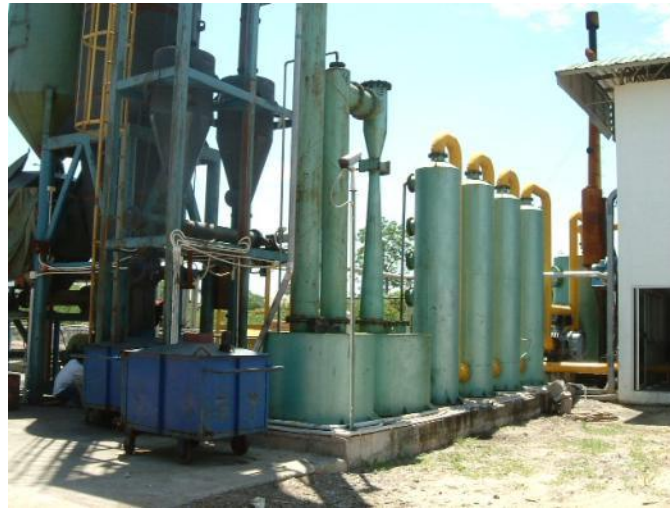
Gas cleaning system
