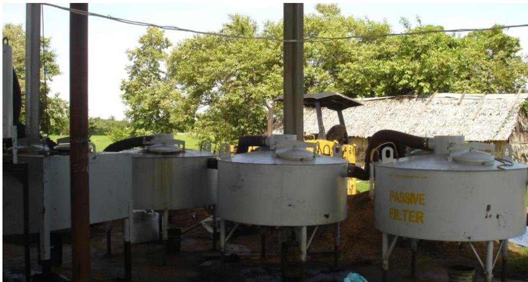
A series of gas cleaning equipment
