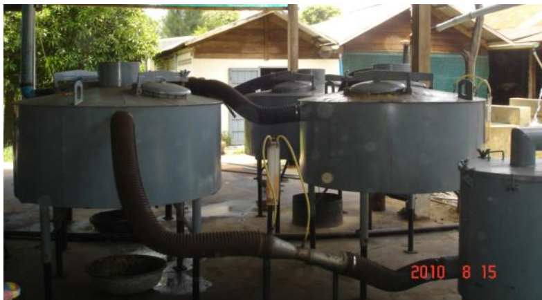
A series of gas cleaning equipments
