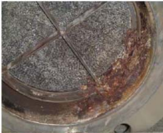
Figure 7-9: Functional impairment of the oxidation catalyst due to condensate failure [55]
