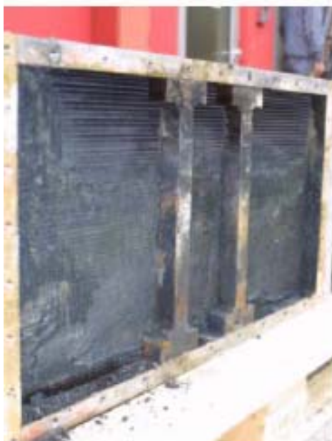
Figure 7-7: Clogging of the outlet side of the intercooler [55]
