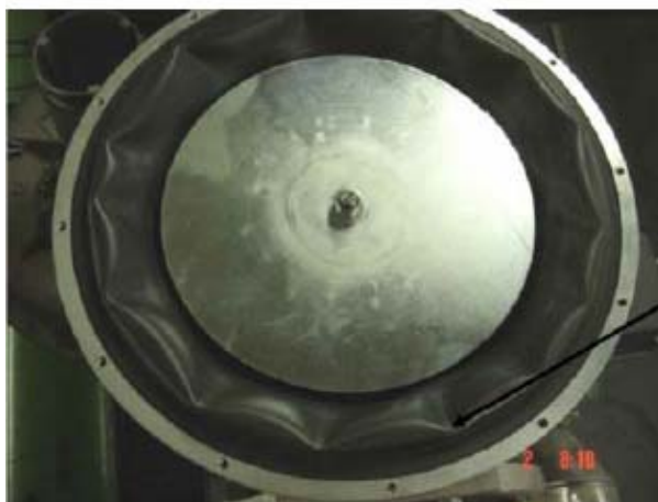
Figure 7-4: Swollen synthetic membrane in the gas control system of the Spiez plant [55]
